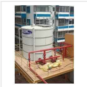
Elevated-Terrace Fire Water Storage Tank
