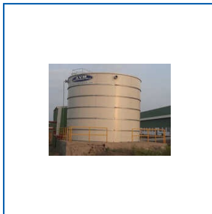
ZINC ALUMINIUM INDUSTRIAL FIRE WATER TANK
