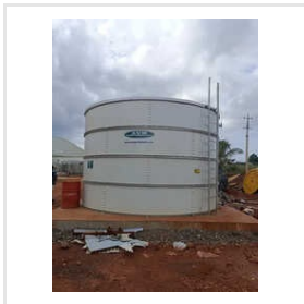
10000L Raw Water Storage Tank
