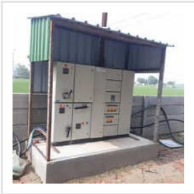
Mushroom Plant Main Control Panel
