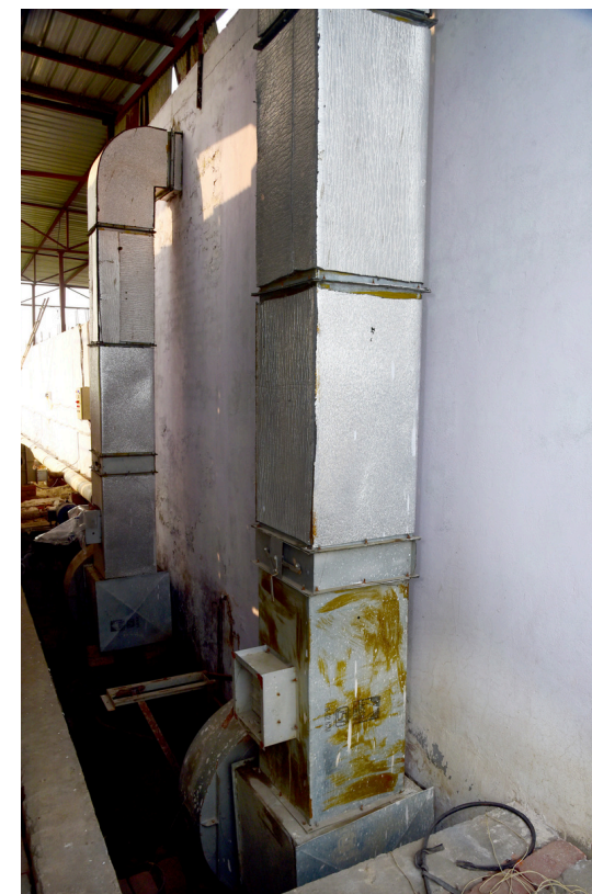
Machines and equipment
