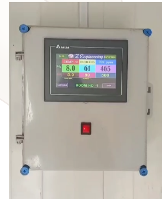
Carbon Dioxide (CO 2 ) System
