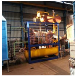
Industrial Modular Process Skids
