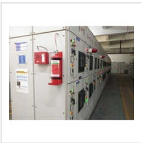
Industrial Fire Suppression System
