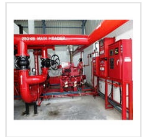
MS Fire Hydrant System
