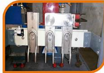
Furnace Selector Switch
