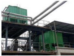
250TR Frp Cooling Towers
