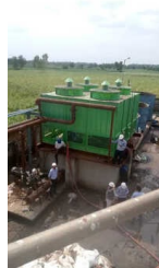
Evaporative Cooling Tower
