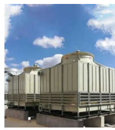
300 TR Industrial Water Cooling Towers
