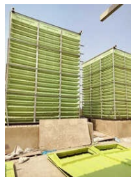
1000TR Natural Draft Cooling Towers
