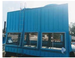
100TR Frp Square Type Cooling Tower
