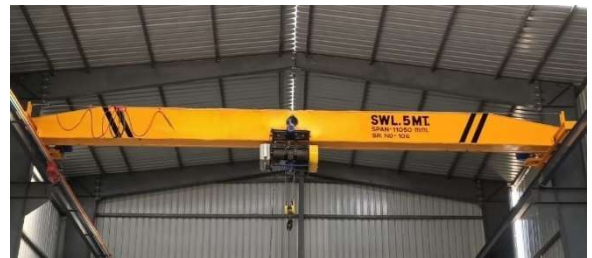
SINGLE GIRDER EOT CRANE
