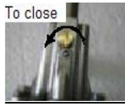
Manual Override "ON" Photo – 2
