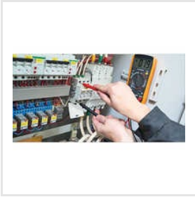
Electrical Control Panel
