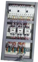
415V VFD Electric Control Panel
