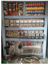
400V PLC Electric Control Panel
