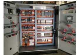
4000A VFD Three Phase Control Panel
