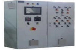
Three Phase Power SPM Control Panel
