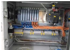
VFD Three Phase Electric Control Panel
