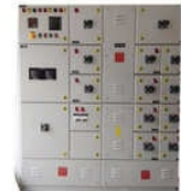
VFD Control Panel
