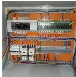
6kW PLC Electric Control Panel
