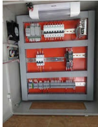
11kV VFD Electric Control Panel
