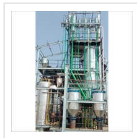
Continous Refining Plant
