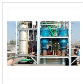
Pre Treatment And Bleaching Plant
