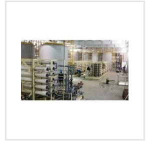
Zero Liquid Discharge System
