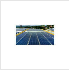
Roof Top Solar Panel
