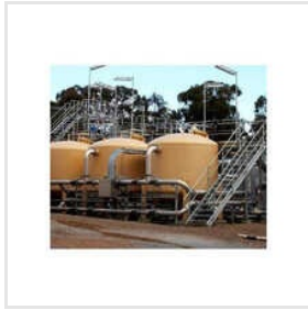
Industrial Effluent Treatment Plant
