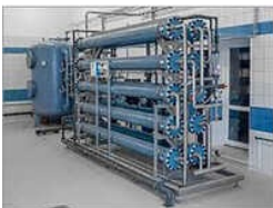
Nano Filtration Plant
