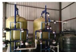
Industrial Water Softener Plant
