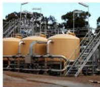
Industrial Effluent Treatment Plant
