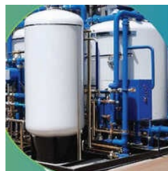
Industrial Water Softener
