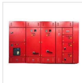
Fire MCC Panel With ACB
