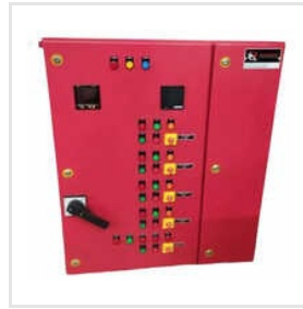
Semi-Automatic MCC Panel
