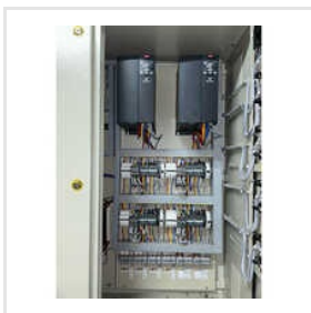
MCC Panel With VFD
