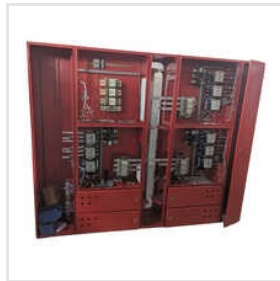
Fire Pump Control Panel
