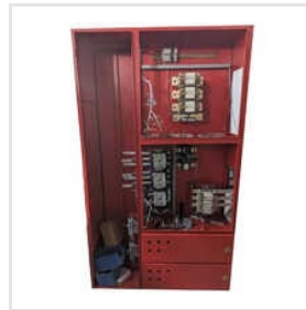
Fire Electrical Control Panel
