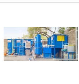
50 KLD Industrial Sewage Treatment
