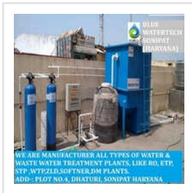
Fully Automatic MBBR Domestic STP
