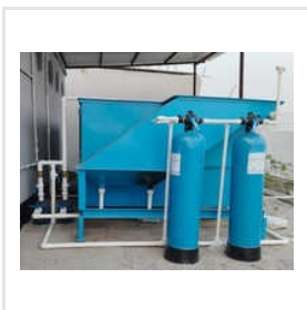
150 KLD Industrial Sewage Treatment
