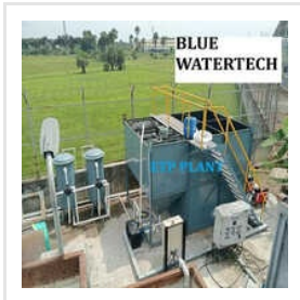
Pharmaceutical 25 KLD Effluent Treatment
