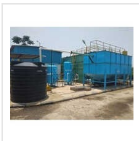
1000 KLD Domestic Sewage Treatment
