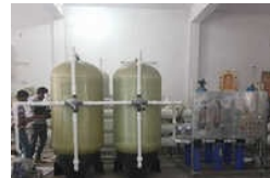
1500 LPH Industrial Reverse Osmosis Plant
