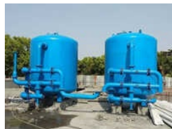
1000 LPH Water Treatment Plants
