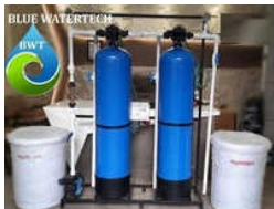
DM Water Plant
