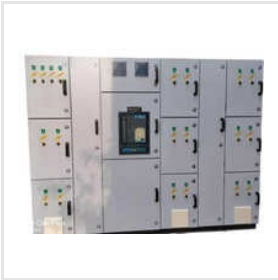
5000amp Automatic Control Panel
