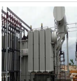
1000 Kva Three Phase Power Transformer
