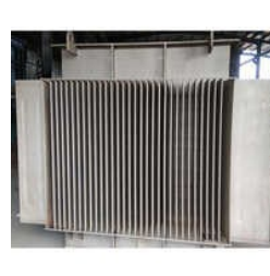
1000 Kva Three Phase Power Transformer
