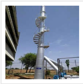
Aluminium Melting Furnace
