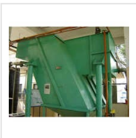
Tube Settler With APC System
