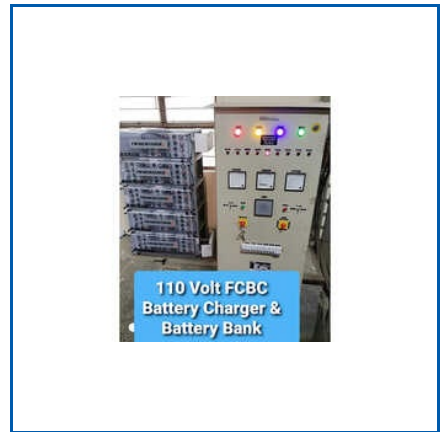
110V FCBC BATTERY CHARGER AND BATTERY BANK
