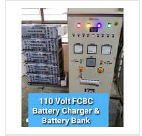
110V FCBC Battery Charger And Battery
