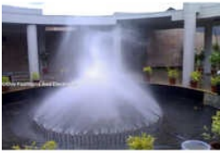
Fog Jet Nozzles Fountain
