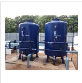
Pressure Sand Filters
