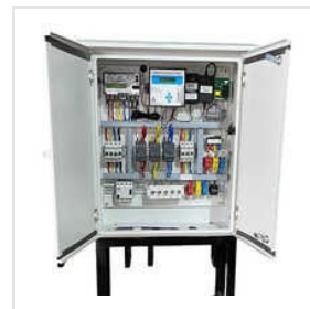
Street Light Control Panel
