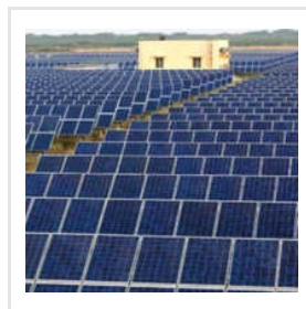
Tata Solar Power Plants
