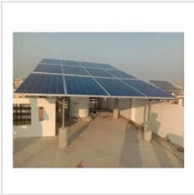
10 KW Hybrid Power Solar System
