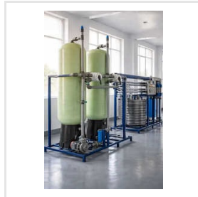
Industrial Pure RO Water Plant
