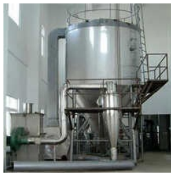
Effluent Spray Dryer Plant
