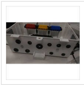
Meter Connection Box
