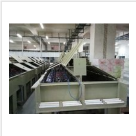
PP Tub For Battery Charging Tank
