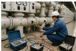
Substation Testing Equipment
