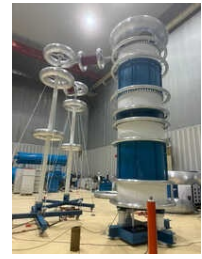
High Voltage Testing Transformer
