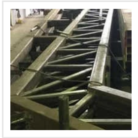
Stainless Steel Trusses
