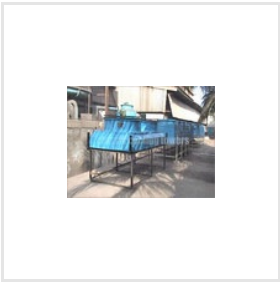
Dry Cooling Towers
