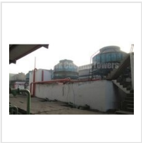
Ajman Shopping Mall Cooling Tower
