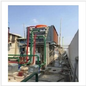
Adiabatic Dry Cooling Towers
