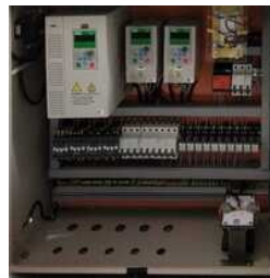
EOT Crane Control Panel
