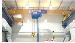
Single Girder Electric Overhead Eot Crane
