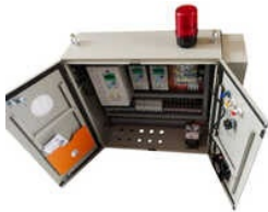
Industrial EOT Crane Control Panel
