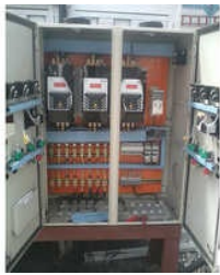
Electric Control Panel
