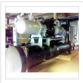
Commercial AC Plant Maintenance Services
