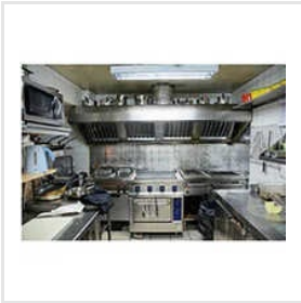
Kitchen Ventilation System
