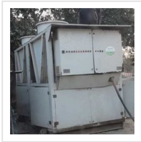
Air Cooled Chiller Plant Maintenance Services
