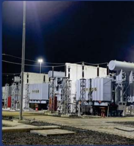
SUBSTATION (AIS & GIS UPTO 400KV)
