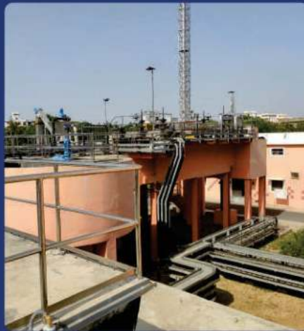
SEWAGE TREATMENT PLANT
