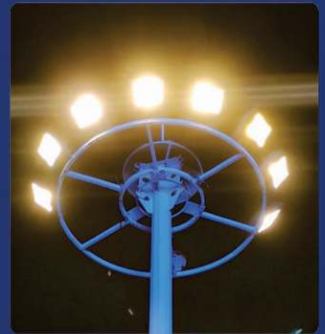
EXTERNAL LIGHTING (HIGH MAST)
