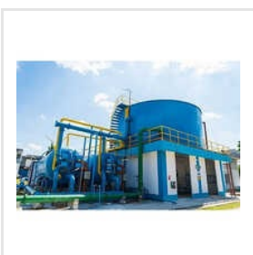
Industrial Water Treatment Plant
