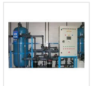
Grey Water Treatment Plant
