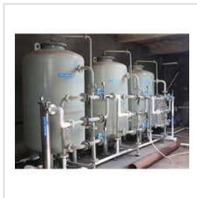
Water Softener Plant
