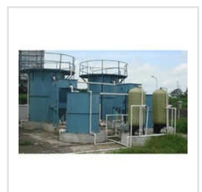
Domestic Sewage Treatment Plant
