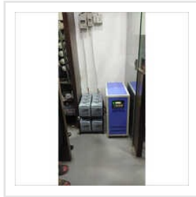
10 KVA Single Phase On Line UPS
