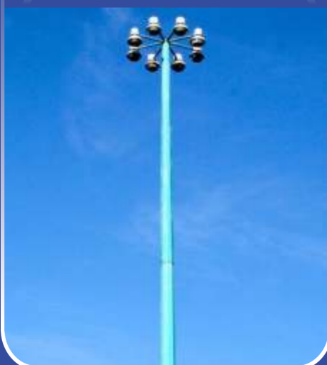
High Mast Pole
