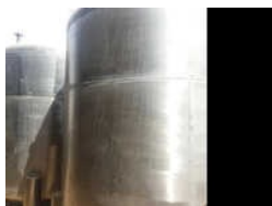
Oil Storage Tanks
