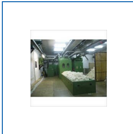
BLOW ROOM LINE
