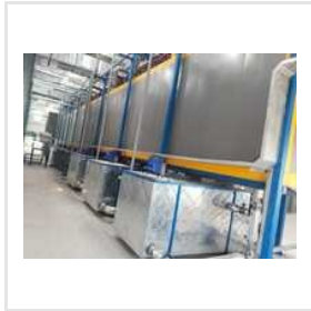
Spray Pre-Treatment Line
