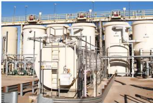
a structure for Application - Reaction Tank
