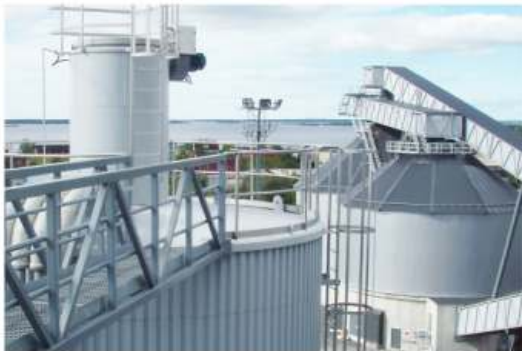
a structure for Application - Ash Handling Plant
