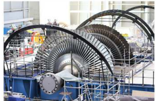
a structure for Application - Steam Turbine
