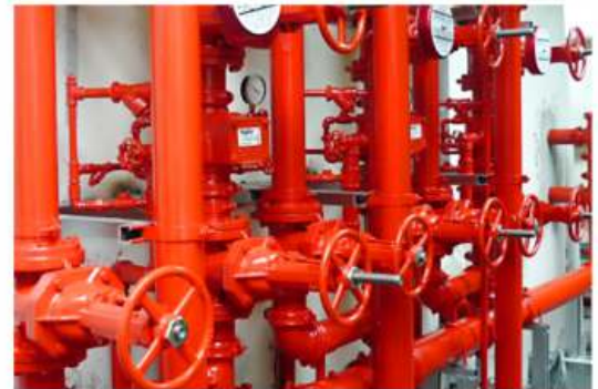
a structure for Application - Fire Fighting
