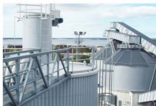
a structure for Application - Ash Handling Plant
