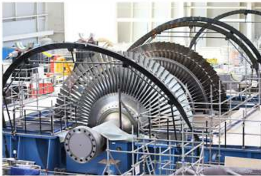
a structure for Application - Steam Turbine
