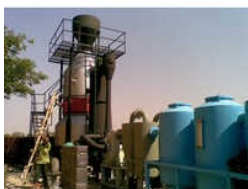
Fuel & Ash Handling System For Gasifiers
