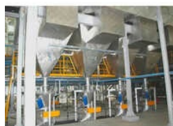
Pneumatic Ash Handling System
