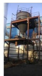
100kg Solid Waste Compost Plant
