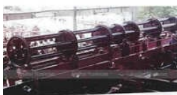
Coal Crushing Plant
