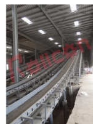
Coal Handling System For Gasification Power
