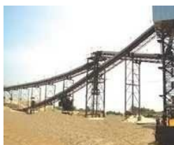
Bagasse Handling System
