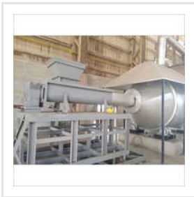
Lead Recycling Plant With Auto Loader
