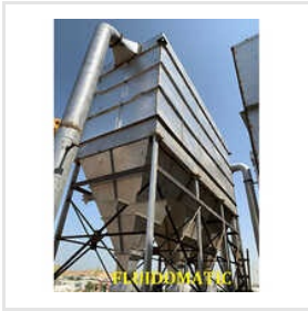
Air Pollution Control System Bag House
