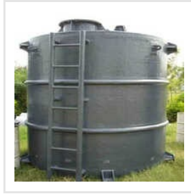
FRP Bottom Storage Tank
