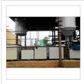
Batch Neutralizing Plant
