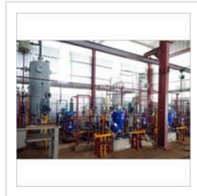
Oil Neutralizer Plant
