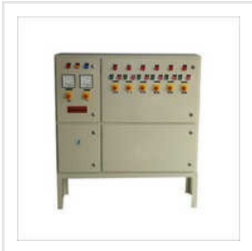
APF Control Panel
