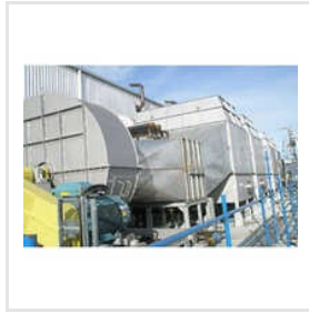
Waste Heat Recovery System
